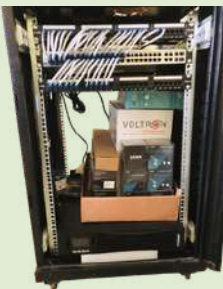
Network Rac with Switch, UPS and Server
